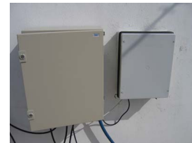
Fig. 5. Core mesh node (left) with EMF monitoring node (right)
