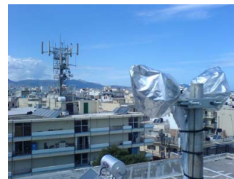
Fig. 6. The EMF node opposite of the antenna tower
